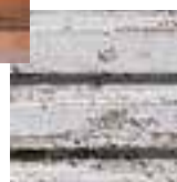
Peeling paint on wood dutchlap
